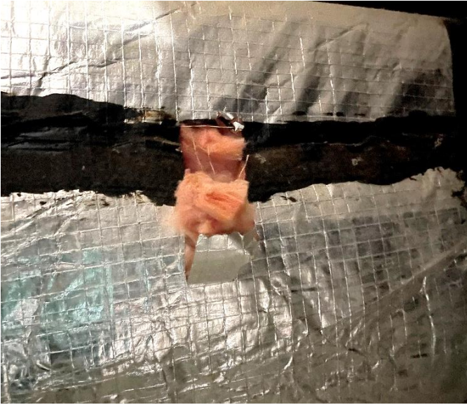
Typical Asbestos Containing Black Mastic on HVAC
