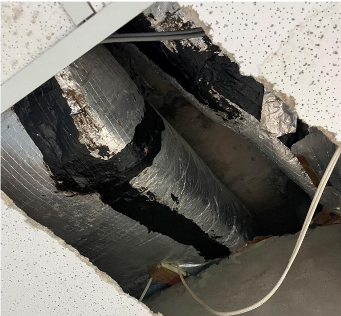
Typical Asbestos Containing Black Mastic on HVAC
