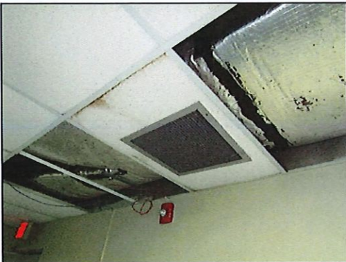
External Clinics Asbestos containing a/c ductwork mastics
