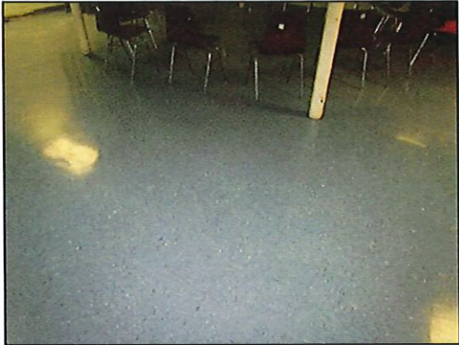
Administration Waiting Area Asbestos containing blue floor vinyl tiles 12"x12" & associated mastics
