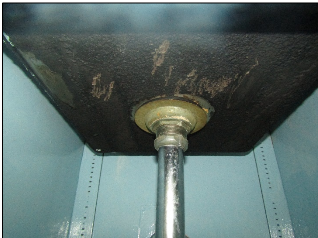
Ward B Asbestos-containing under sink mastic.
