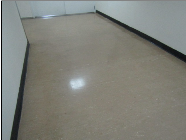
Ward B Asbestos-containing floor covering.
