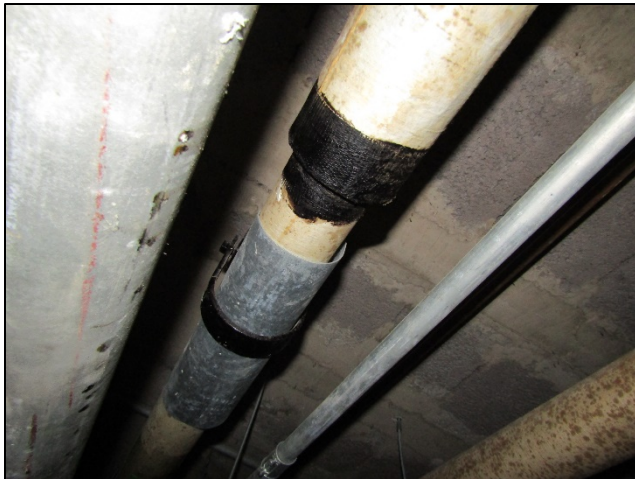
Ward B Asbestos-containing mastic on TSI joint.
