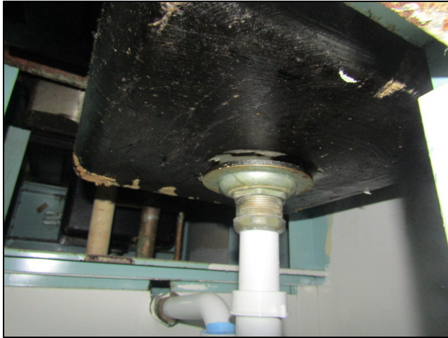
Ward B Asbestos-containing under sink mastic.
