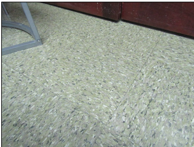
Ward B Asbestos-containing green vinyl tiles (12x12) & associated mastic.
