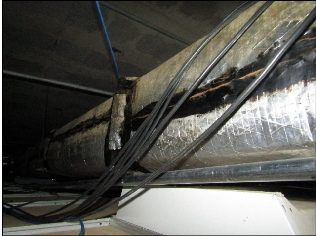
Ward B Asbestos-containing A/C duct mastic.
