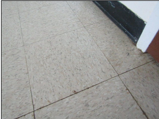
Ward B Asbestos-containing cream vinyl tiles (12x12) & associated mastic.
