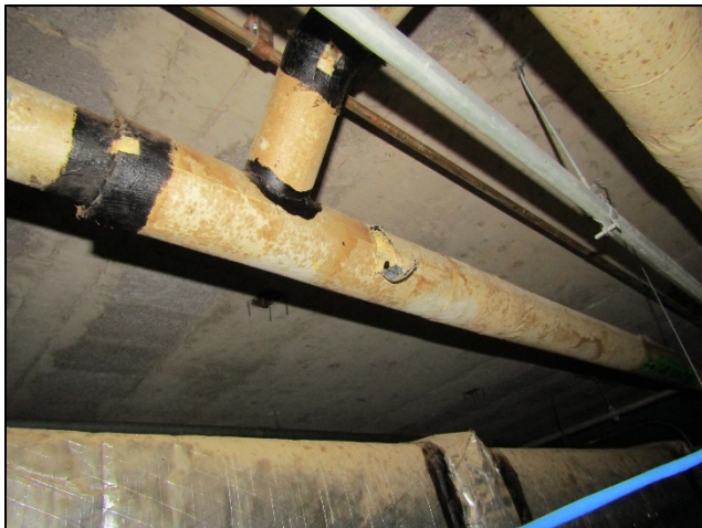
Ward B Asbestos-containing mastic on TSI elbow.
