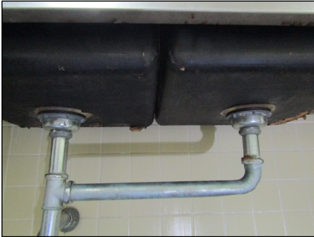
Delivery Room Areas Asbestos-containing under sink mastic.
