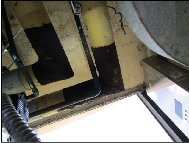
Ward B Asbestos-containing mastic on TSI elbow.
