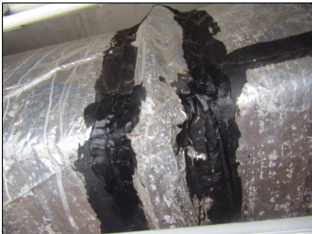
Ward B Asbestos-containing A/C duct mastic.
