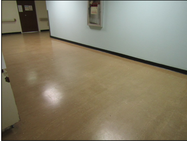
Ward B Asbestos-containing floor covering.
