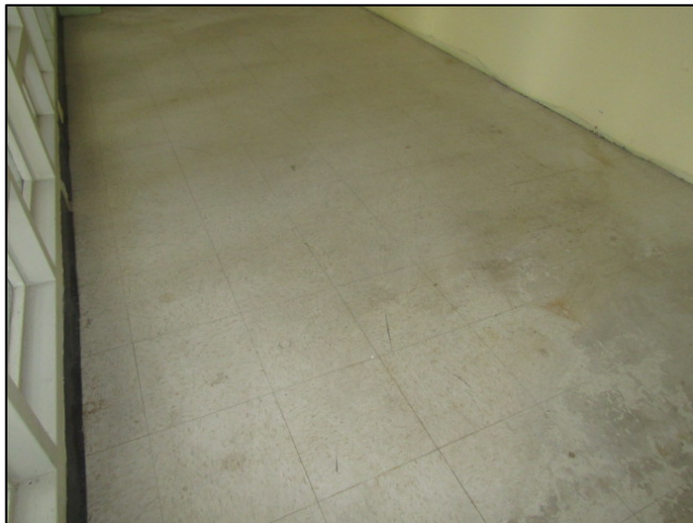
Ward B Asbestos-containing light cream vinyl tiles (12x12) & associated mastic.
