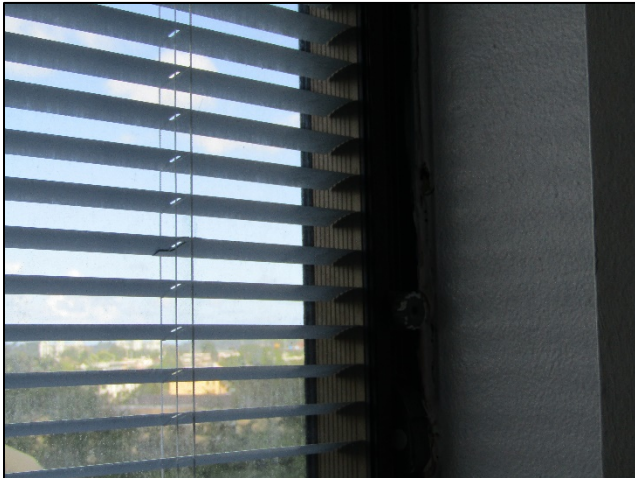
Ward B Asbestos-containing window caulking.
