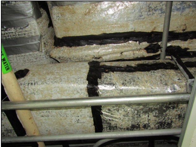
Delivery Room Areas Asbestos-containing A/C duct mastic.
