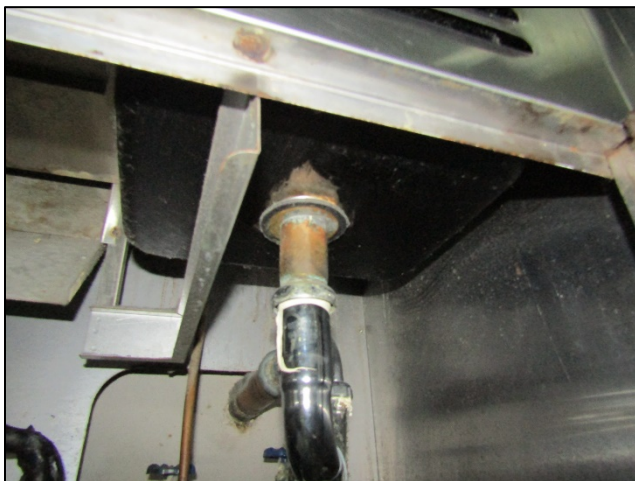
Delivery Room Areas Asbestos-containing under sink mastic.
