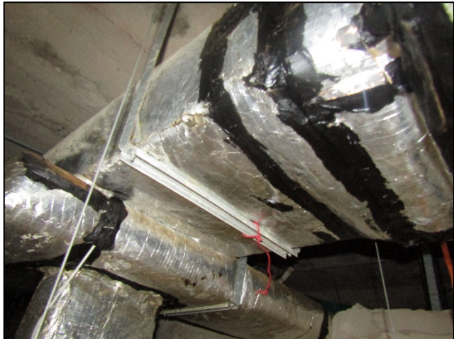
Ward B Asbestos-containing A/C duct mastic.
