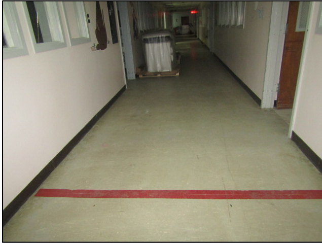
Delivery Room Areas Asbestos-containing gray floor covering.
