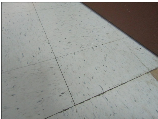
Ward B Asbestos-containing white vinyl tiles (12x12) & associated mastic.
