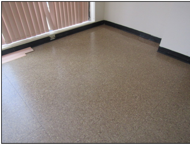
Ward B Asbestos-containing brown vinyl tiles (12x12) & associated mastic.
