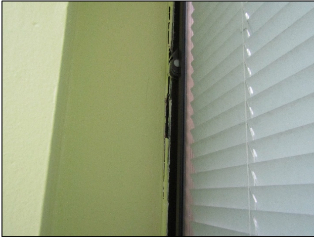
Ward B Asbestos-containing window caulking.
