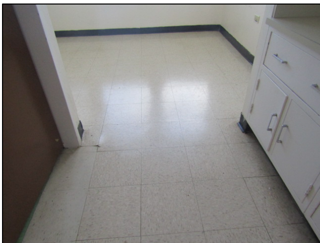
Ward B Asbestos-containing cream vinyl tiles (12x12) & associated mastic.
